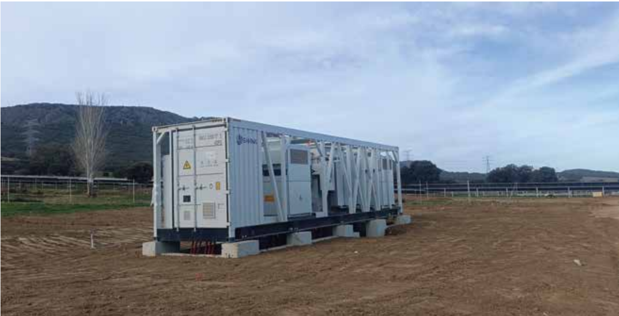
350MW PV Plant, Spain
