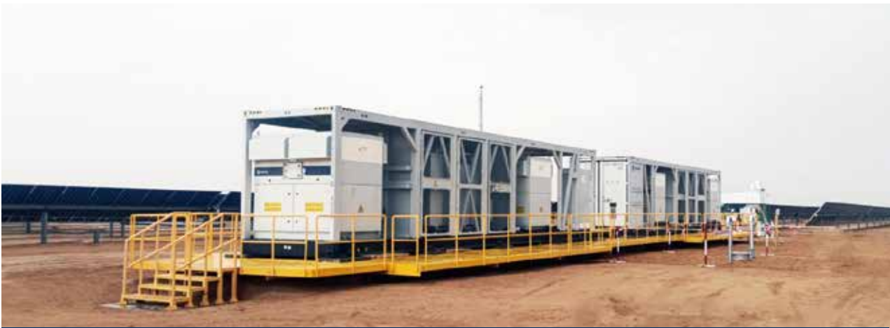
760MW PV Plant, Saudi Arabia
