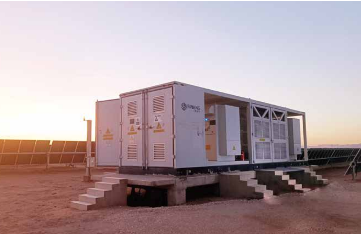
24MW PV Plant, Jordan
