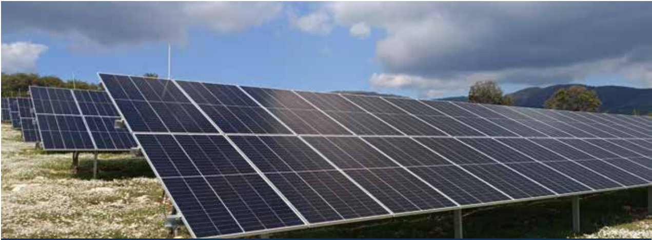
13.75MW PV Plant, Greece
